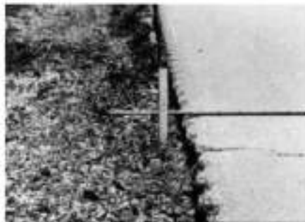
Figura 11.24 Desnivel carril -berma – Severidad alta
