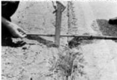
Figura 11.23 Desnivel carril -berma – Severidad media
