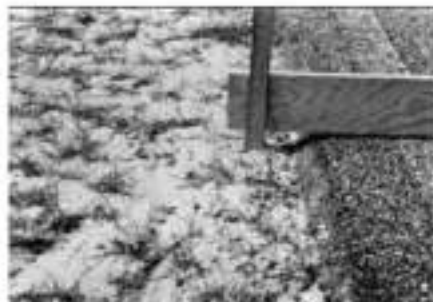
Figura 11.22 Desnivel carril -berma – Severidad baja
